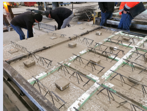
Embedded concrete sprinkler holders. On site, the rest of the pipework and sprinkler fittings are connected.
