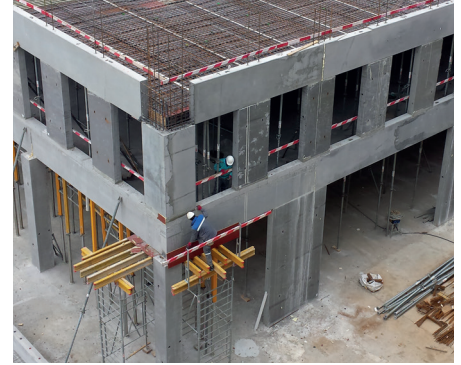
Belgium - Concrete core activation
