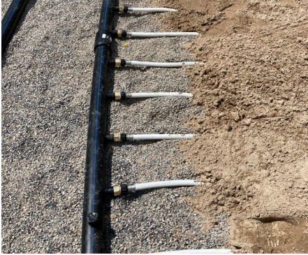
Andorra - Soccer field heating
