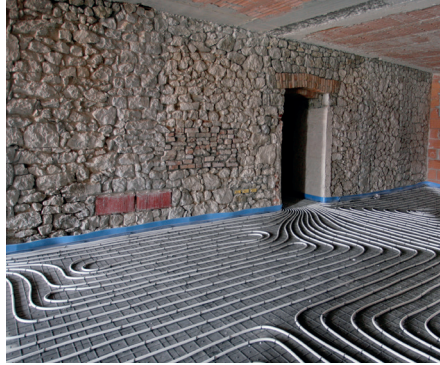
Italy - Floor heating in castle
