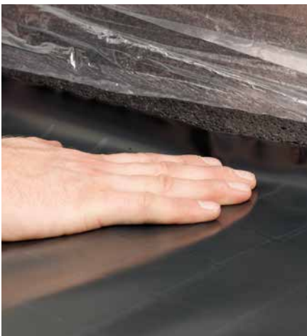
The PE sheeting is installed on the walls: when doing this, there must be a good overlap with the PE flap of the edge insulation.
