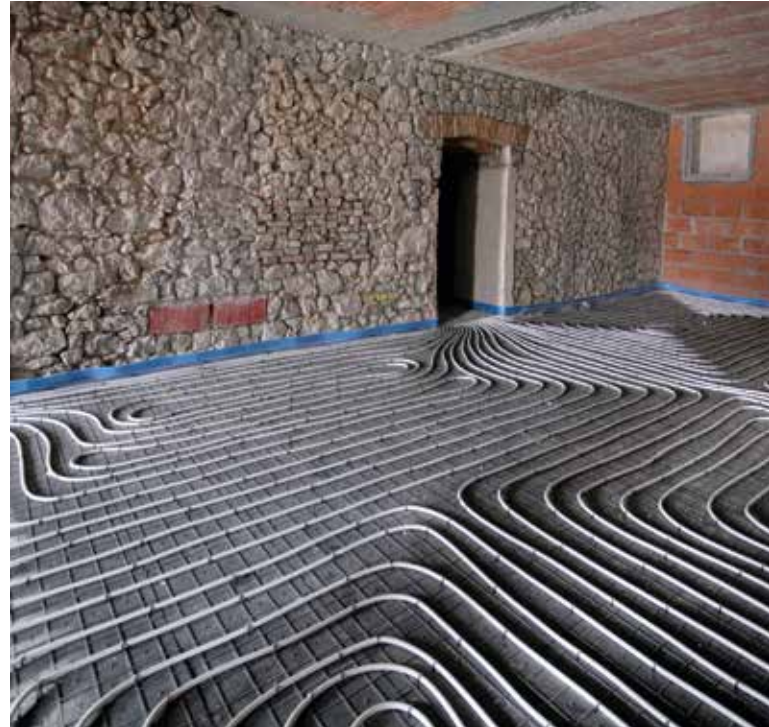
Castle, Italy ▲ Underfloor heating and cooling
