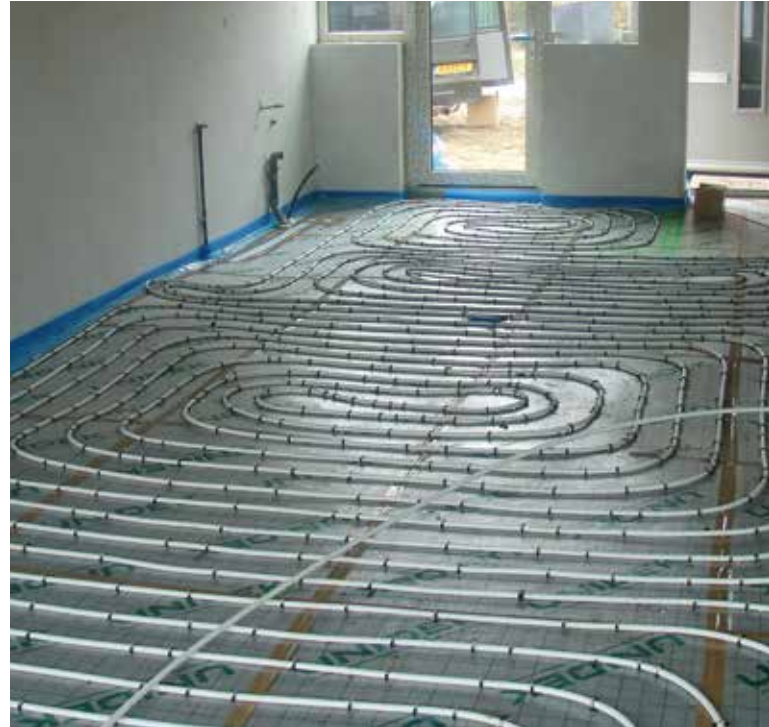
Schouten, The Netherlands ▲ Underfloor heating
