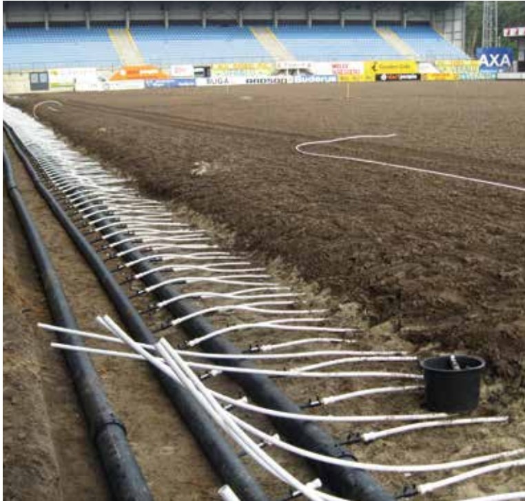
▲ Football stadium, Westerlo, Belgium Football field heating
