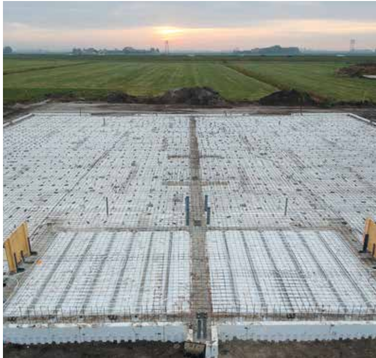
▲ Project Lemmer, Friesland, The Netherlands Underfloor heating
