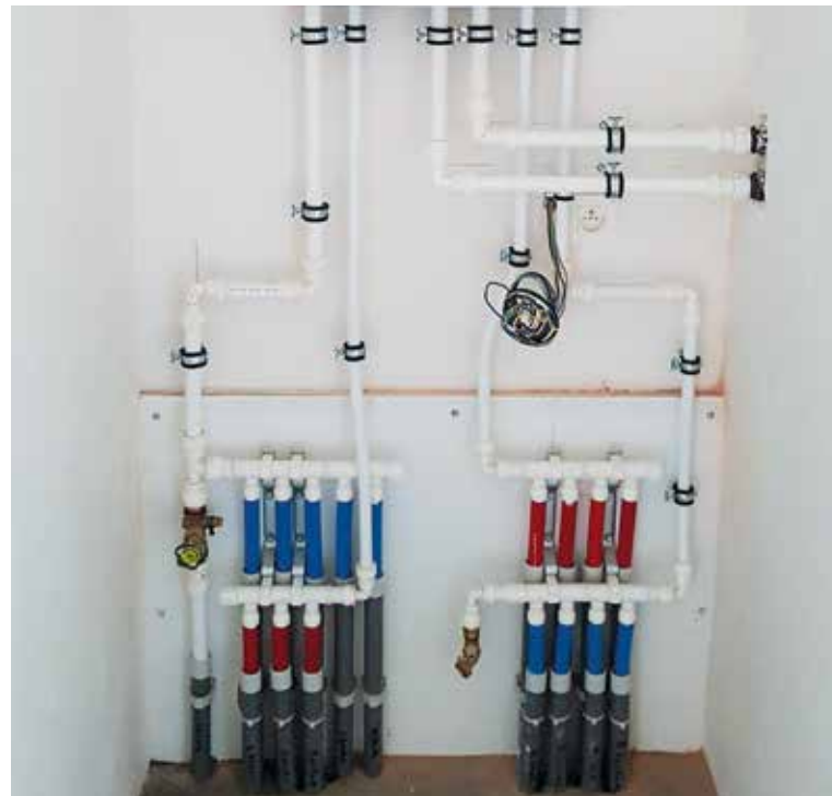
Apartments, Belgium ▲ Henco Vision installation for sanitary
