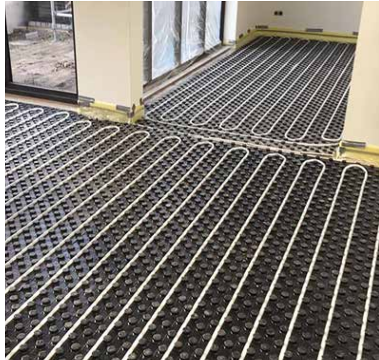
Breda, The Netherlands ▲ Underfloor heating
