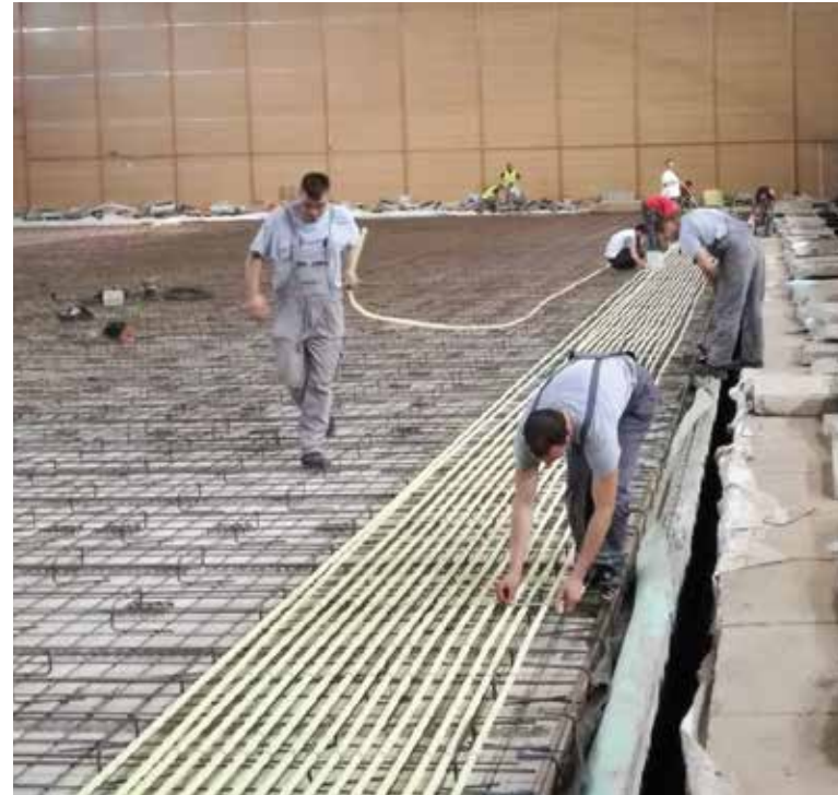
▲ Rink Stadium, Zagreb, Croatia Cooling system for indoor ice skating ring
